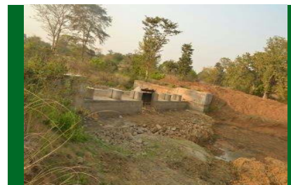
Sluice Valve For the Check Dam
